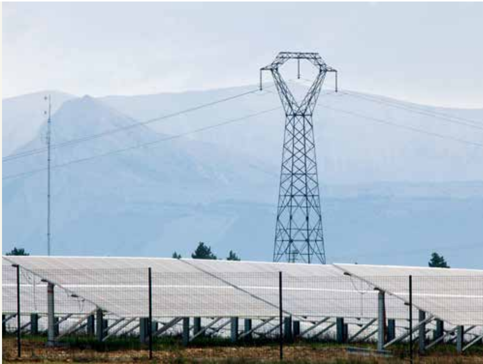
◀ Connecting new production facilities may require improvements to be made to the public electricity network. . View of “Les Mées” photovoltaic farm in Alpes-du-Sud.
